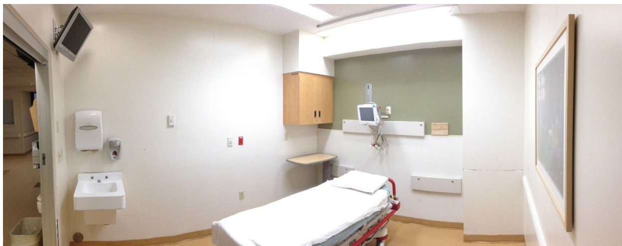
A moderately “Psych Safe” emergency department exam room. Prison grade sink, secure flip down covers to conceal power, data and medical gas outlets.
